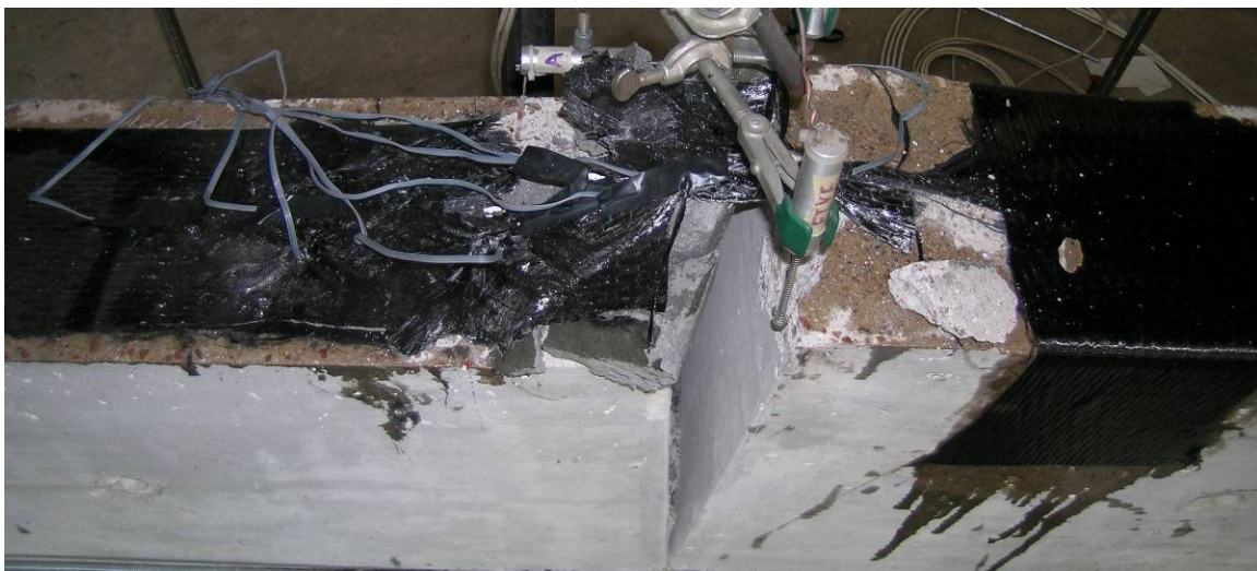
After Testing: Failure by FRP Fracture
