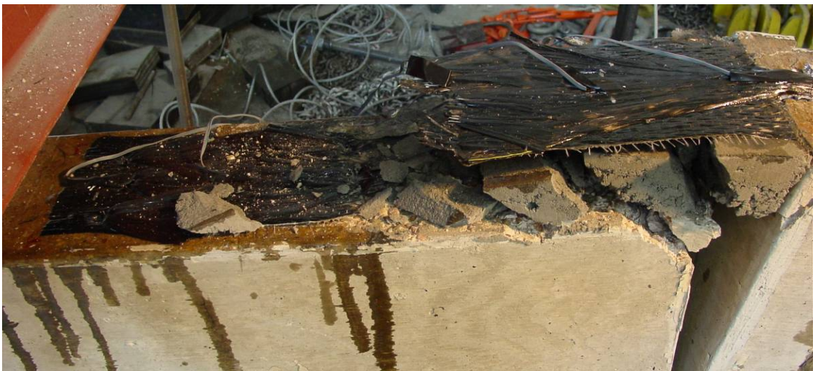
After Testing: Failure by FRP fracture
