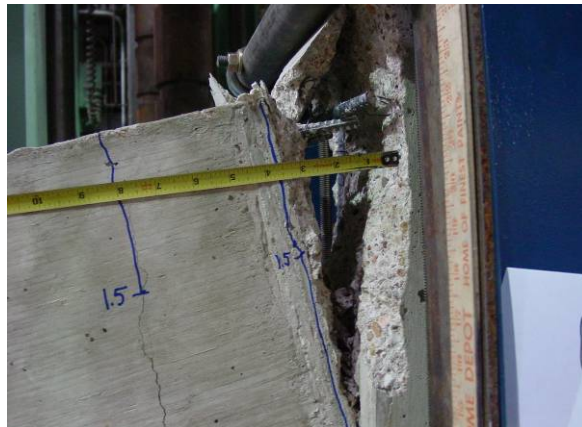
Wide crack at column
