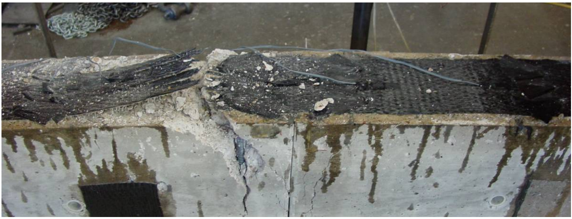
After Testing: Failure by FRP fracture
