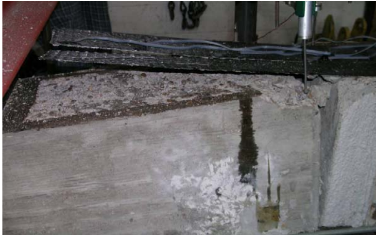
Figure 4-12 Debonding of CFRP
