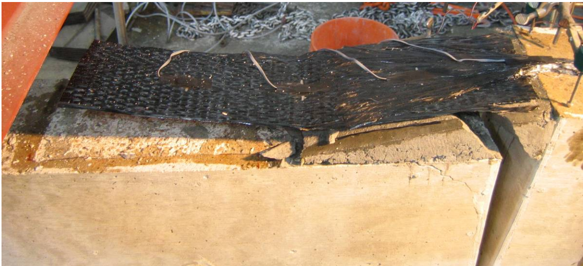
After Testing: Failure by debonding
