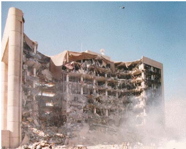
Figure 2-2 Collapse of Murrah building [Crawford, 2002]
