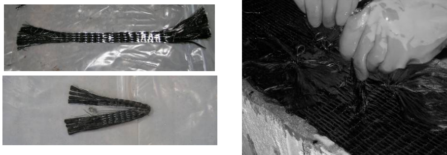
Figure 3-20 Strips of CFRP used to form anchor and inserting anchor into predrilled hole
