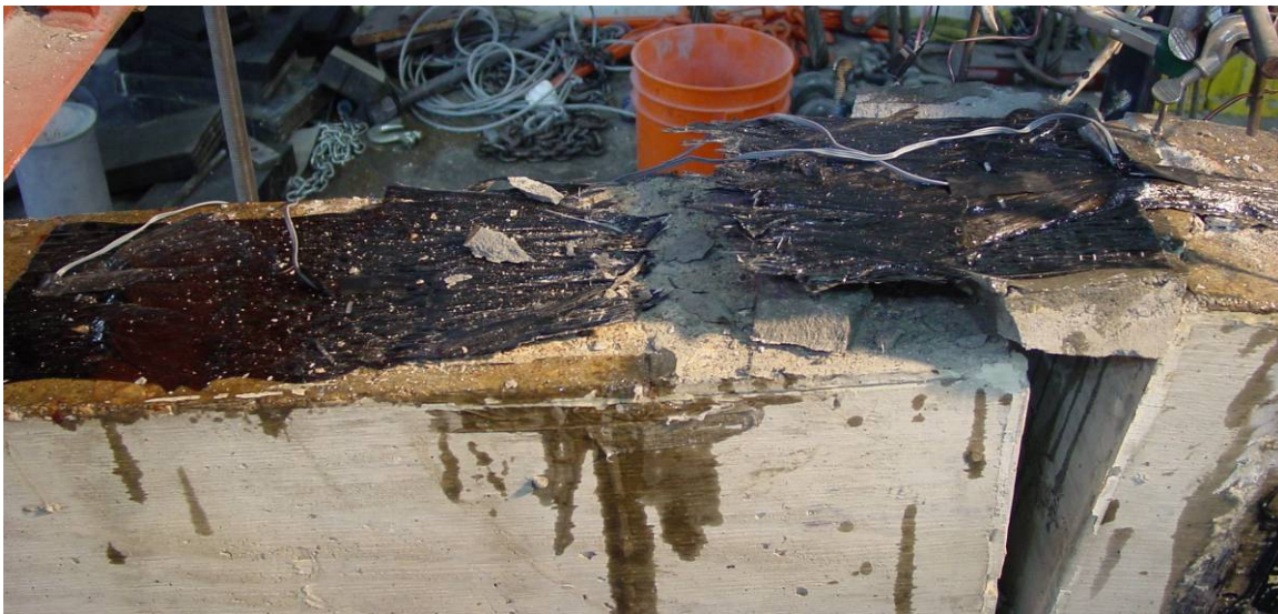
After Testing: Failure by FRP fracture
