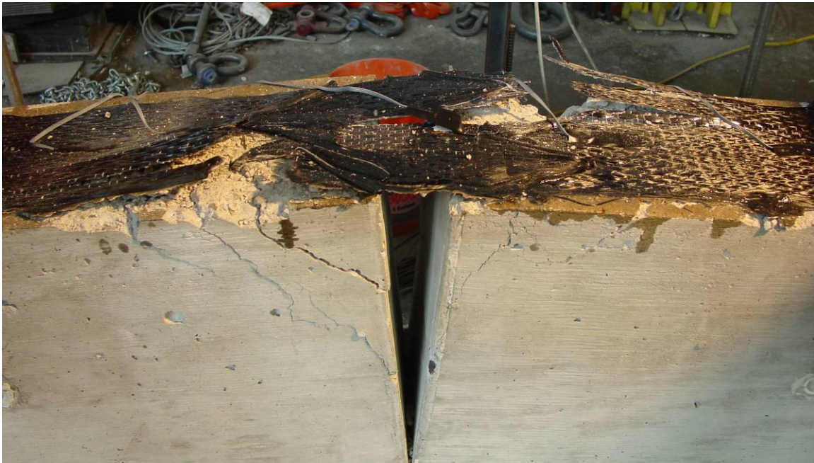
Figure 4-18 Failure by FRP fracture of retrofit with two anchors per row (00-4s2)
