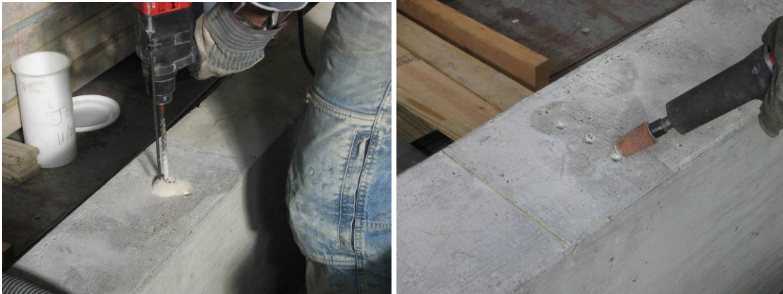
Figure 3-32 Drilling hole in concrete and rounding over edges (courtesy of Insung Kim)
