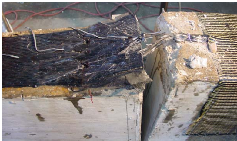
Figure 4-25 Fracture of CFRP at top of transition slope in test 22-6s1
