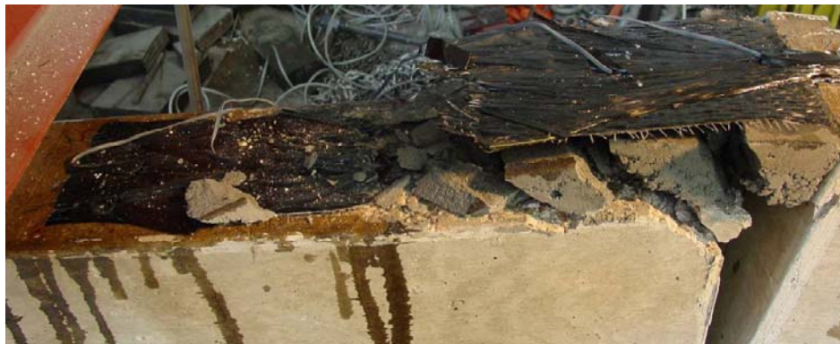
Figure 4-32 Failure of 43-6s1 with 3" height difference
