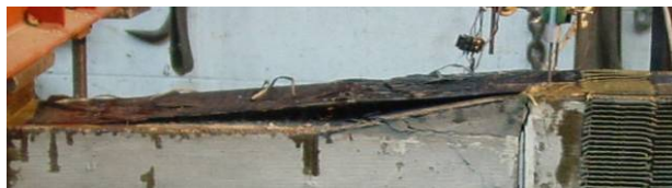
Fracture first row of anchors
